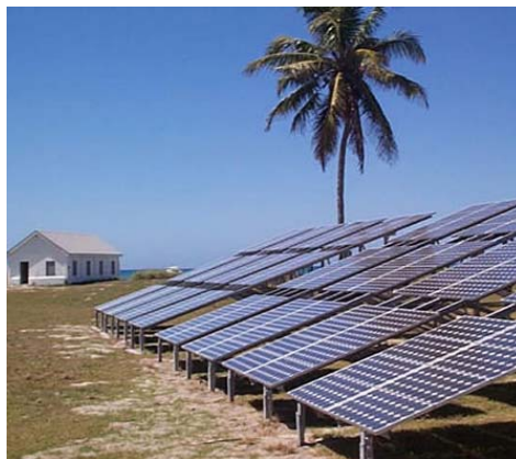
This Dry Tortugas National Park system has withstood hurricanes and years of salt water spray and continues to power employee housing and potable water production.
