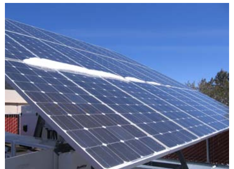
This Solar PV system at a BTS site in a mountainous region in California is subjected to snow and extreme temperatures.
